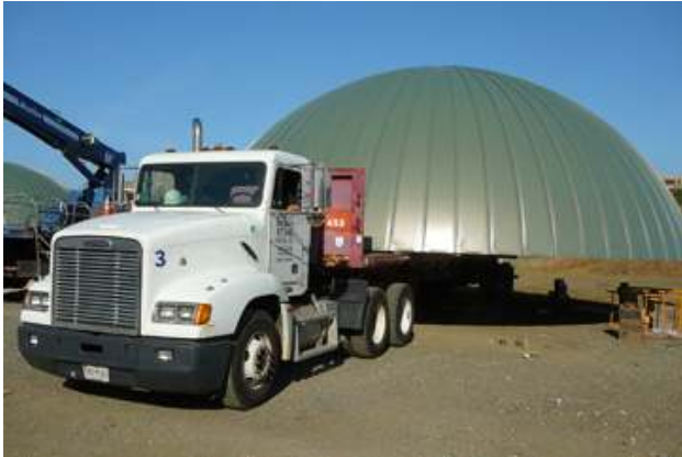
The dome is supported with structural steel reinforcement on the inside, engineered to withstand 90 mph winds, as well as transport to the site. No highway travel was required in this installation.
