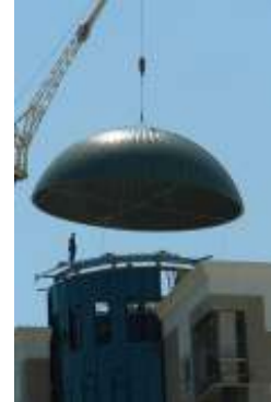
An ironworker, with full fall protection, guides the crane operator by 2-way radio.
