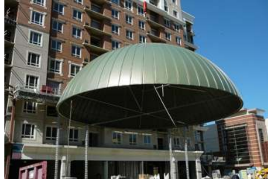
A dome is lifted by crane from the truck, on its way to the roof structure. The domes were tested for wind resistance, and found to be very aerodynamic, and not susceptible to minor swirling winds.
