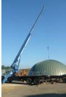
A finished dome is loaded on a flatbed truck for delivery to the nearby lift site.
