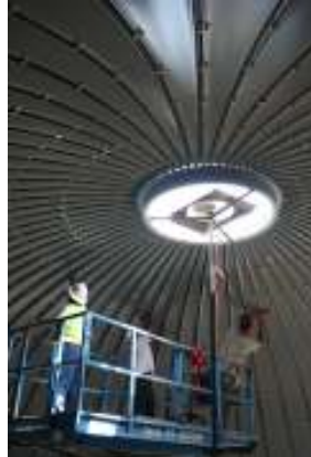
Workers tighten fasteners from the inside. No workers are exposed to working on the exterior.
