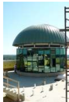
The dome in place. Each dome is finished with concrete cornice work, somewhat like crown molding.
