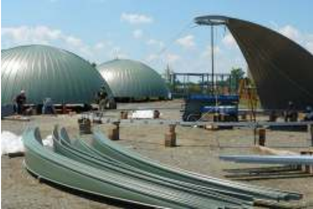
Dome roofs, destined for placement 150' high, are assembled on the ground to help maximize safety and speed assembly time. Three domes are each 37' 9" in diameter.
