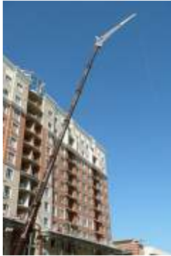
The domes weigh 4,200 pounds each. In terms of crane lifting, this represents a relatively light load.
