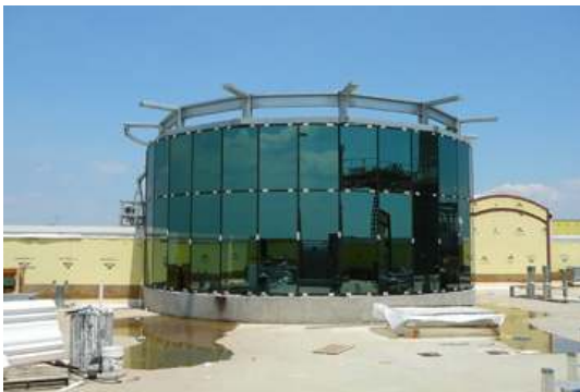
One of three structures where a 37' 9" Lancaster Dome was placed atop the new condominium building.
